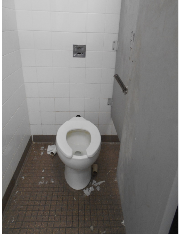
Lincoln – bathroom stool (there are 5 stalls)
