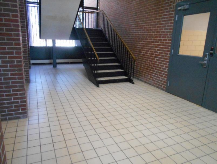
School – foyer between school and gym (there is also an area about 6 ft wide between doors at the bottom of this picture)
